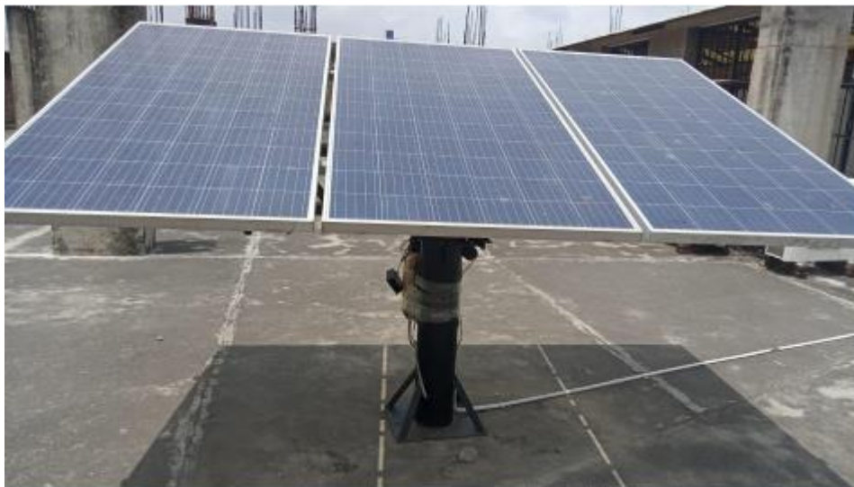
Rooftop solar power plant
