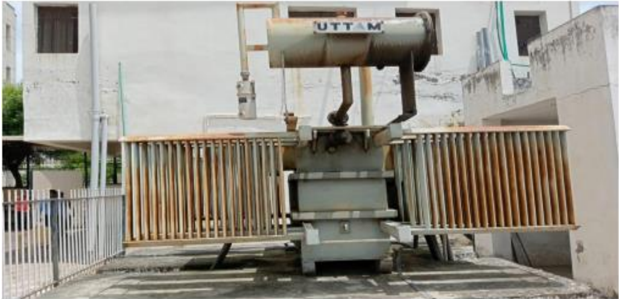
Distribution transformer of 750KVA
