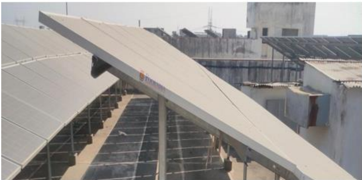
Solar Power Plant on terrace
